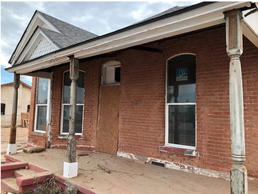
10/31/2017 – Front porch view, looking southeast from neighbor's driveway
