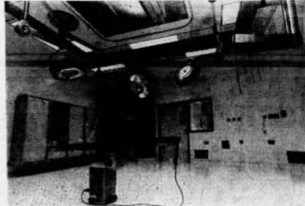
Operating room contains table (foreground) flanked by C-Lockers containing supplies (left wall), electrical outlets that dangle from the ceiling so no one falls over cords, special down-draft air circulation that reduces risk of infection.
