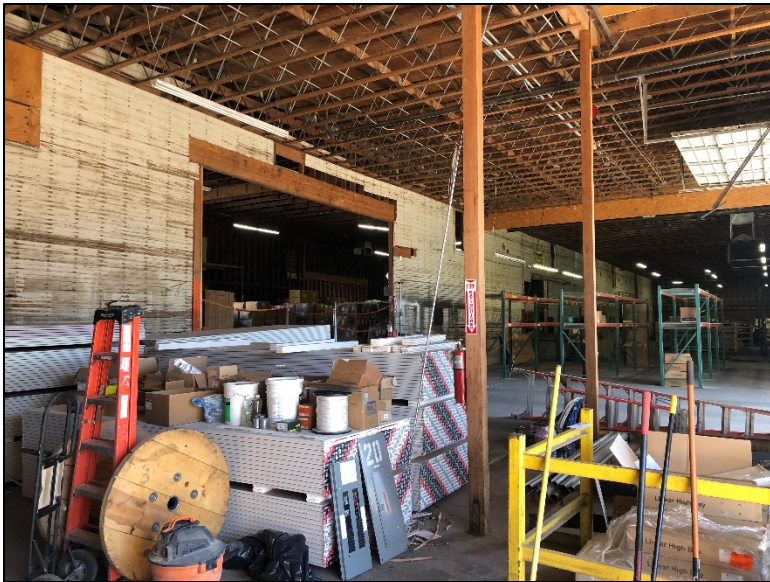
Photo 11. Interior view of nonhistoric metal addition, with encapsulated historic wood frame structure.
