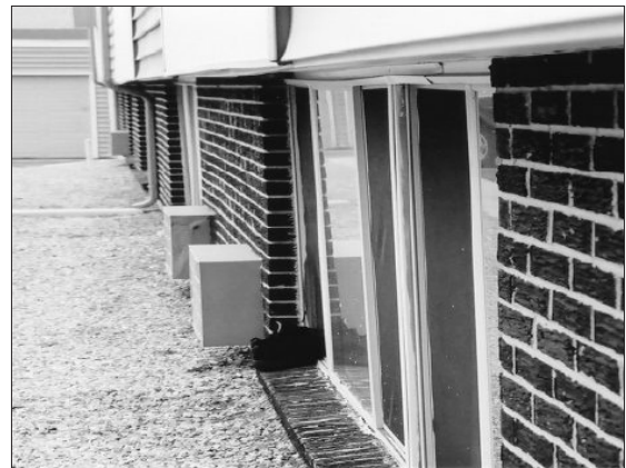
Vinyl window frames are constructed of polyvinyl chloride (PVC), a plastic material that breaks down in direct sunlight. To increase their longevity, vinyl frames include UV light stabilizers to keep them in good condition. However, over time, these windows may begin to lose their color, turn yellowish, or degrade. They are particularly susceptible to warping at high temperatures, as seen in the example above.
