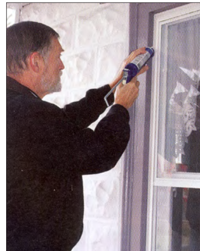
Caulking between exterior window jambs and wall surfaces is recommended to reduce air infiltration.
