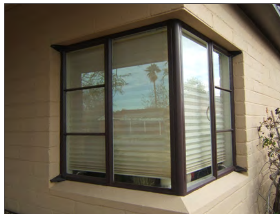
The original glass in this steel casement window (top) was replaced with single-pane hard coat Low-E glass (below).
