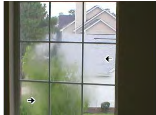
A common problem with dual-pane replacement windows is that the insulating seal will eventually leak and moisture will penetrate between the glass, leaving the window looking foggy. When this happens, the glass—or perhaps the entire window—will need to be replaced again.
