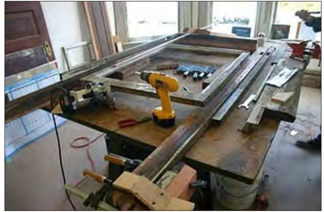
Most wood windows can be repaired. Depending on the condition of the window, it may be necessary to remove the sash and/or the affected parts of the jambs and have a carpenter or woodworking mill repair or reproduce the damaged or missing parts.
