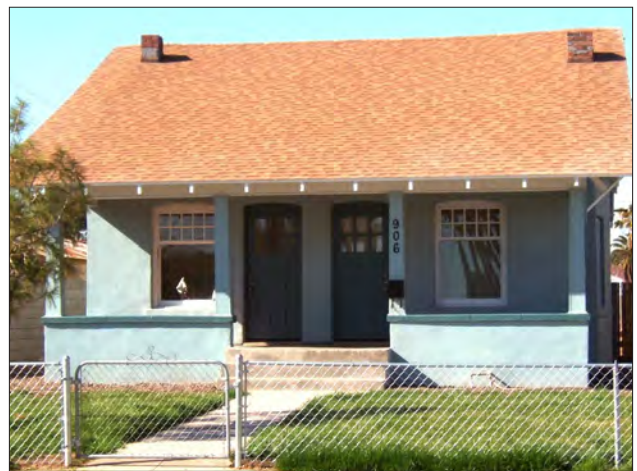
In the example above, the top photo was sufficient pictorial evidence to show that one of the front windows was nonhistoric and that its replacement (shown in bottom photo) should match the window that still remained.
