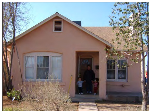
The original wood windows on this house had been replaced with incompatible aluminum sliders, with the openings reduced in size. Fortunately, there was sufficient documentation to replicate the original windows and restore the house back to its historic appearance.
