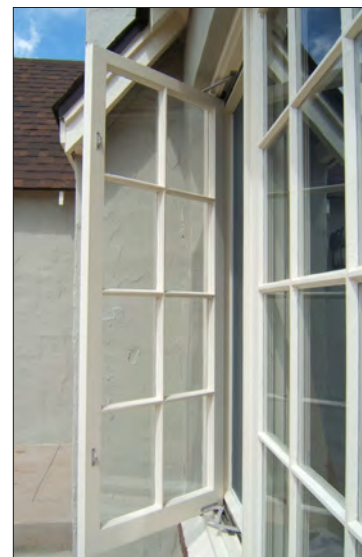
This new wood window utilized the same material as the window it replaced, as well as the same muntin pattern.
