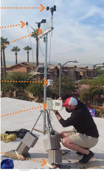
In the photo above, a researcher is making repairs to a weather station on the roof of an apartment building in Phoenix. Did you know there were so many different pieces of equipment involved?
